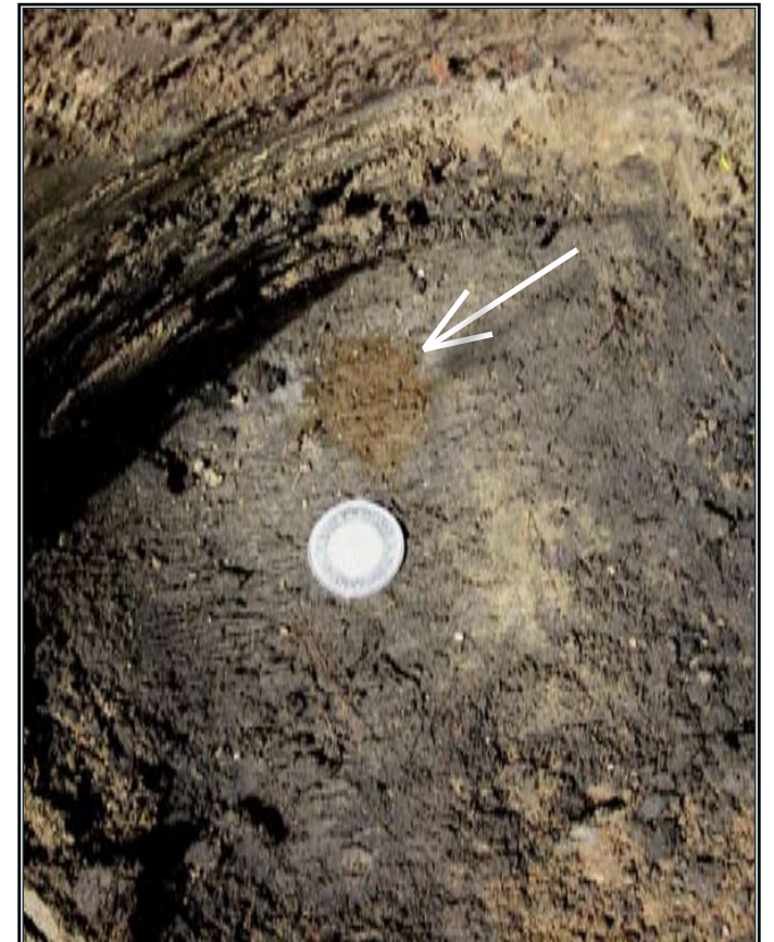
The unmistakable evidence of a rust hole left by the original township monument.
